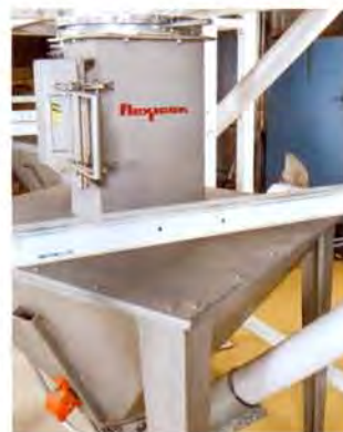
Peanuts are discharged from the bulk bag into the receiving hopper through a manually operated 12 in. (305 mm) diameter iris valve attached to the bag spout.
