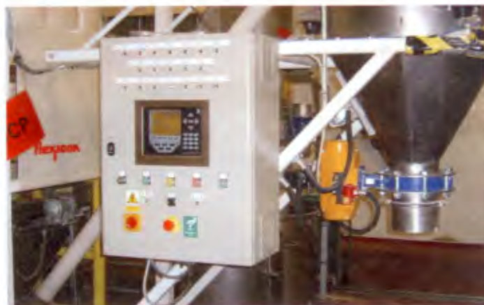
ABOVE: Control system with full function weighing indicator controlling discharge into the weigh hopper.
