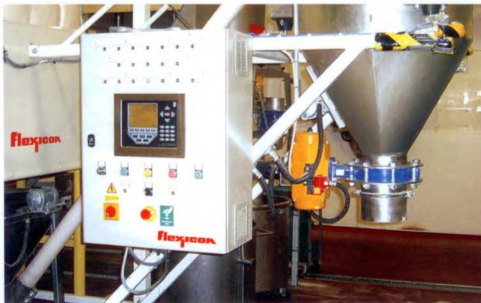
Control system with full function weighing Indicator starts and stops conveyor, and actuates a slide gate.
