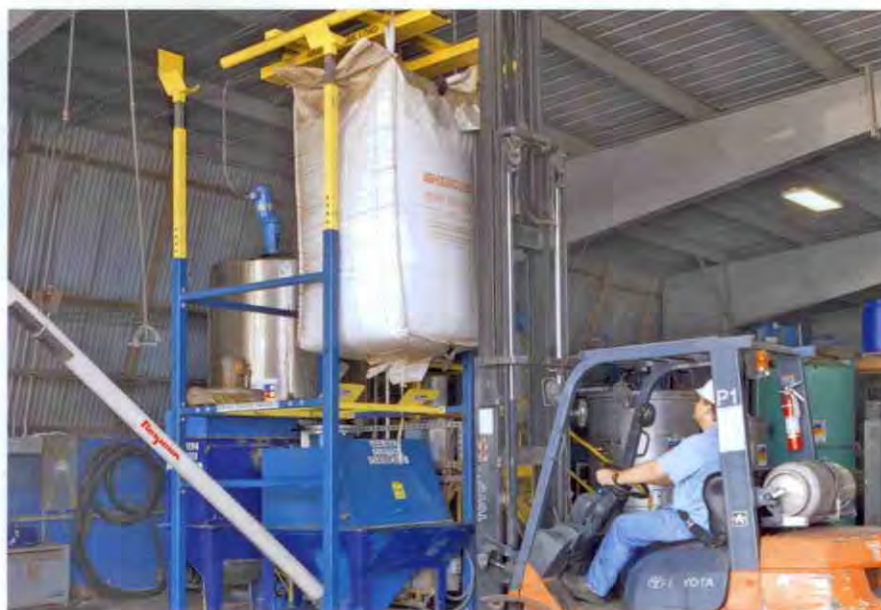
Forklift operator positions bag lifting frame on top of the bulk bag unloader. The 6,7 m long flexible screw conveyor transports resin from the bag dump hopper into a 22 713 ℓ tank.
