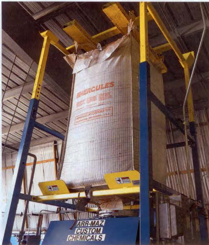
At top of the unloading frame, Pop-Top bag extension devices raise and elongate the bulk bag, promoting flow through the bag spout. At bottom, pneumatically actuated Flow Flexer plates raise and lower opposite bottom sides of the bag, loosening material and directing it through the bag spout.
