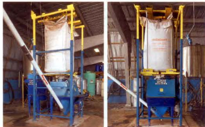
Cradle at top of the bulk bag unloader supports the removable bulk bag lifting frame. An iris valve between the bag spout and manual dumping hood controls the rate at which the bulk resin enters the hopper.
