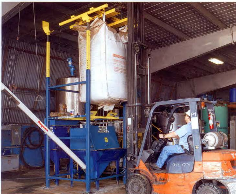
Forklift operator positions bag lifting frame on top of the bulk bag unloader. The 6.7m long flexible screw conveyor transports resin from the bag dump hopper into a 22,713-litre tank.
