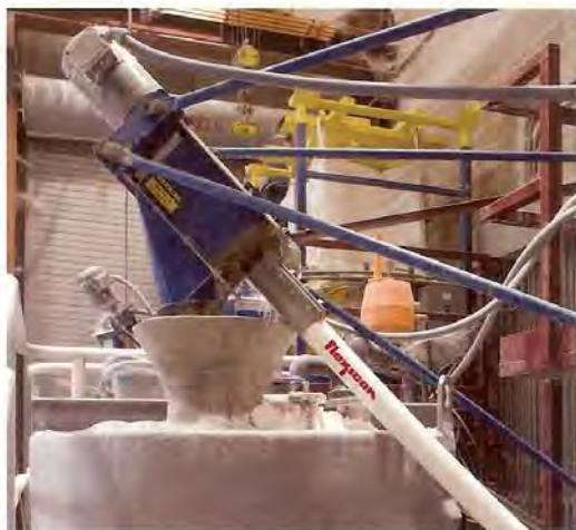
At the flexible screw conveyor's discharge end, DE flows through a transition adapter into the 1136 L tank where the DE is put in suspension with water.
