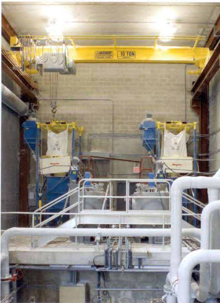
The bridge crane (top yellow beam) and movable hoist allow an operator to easily lift and seat a 900-pound-capacity bulk bag in either discharger.
