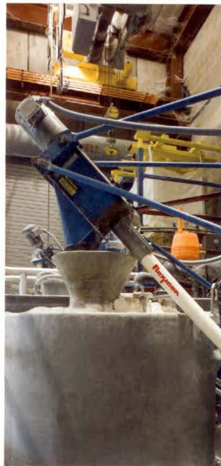
At the flexible screw conveyor's discharge end, DE flows through a transition adapter into the 1136 litre tank where the DE is put in suspension with water.
