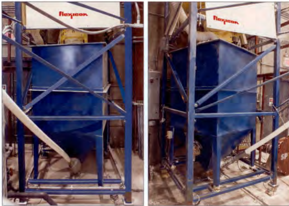
The 1.8-cubic-metre capacity hopper holds the contents of a 408-kilogram bulk bag allowing diatomaceous earth to transfer, unattended, through the flexible screw conveyor to the tank. Load cells under the unloader frame transmit weight loss information to a PLC to achieve accurate batch weight transfer.
