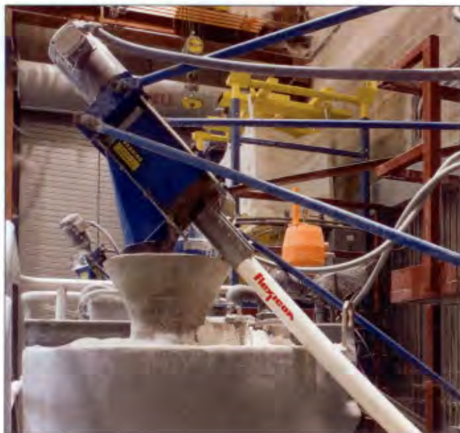
At the flexible screw conveyor's discharge end, diatomaceous earth flows through a transition adapter into the 1136-litre tank where the diatomaceous earth is put in suspension with water.
