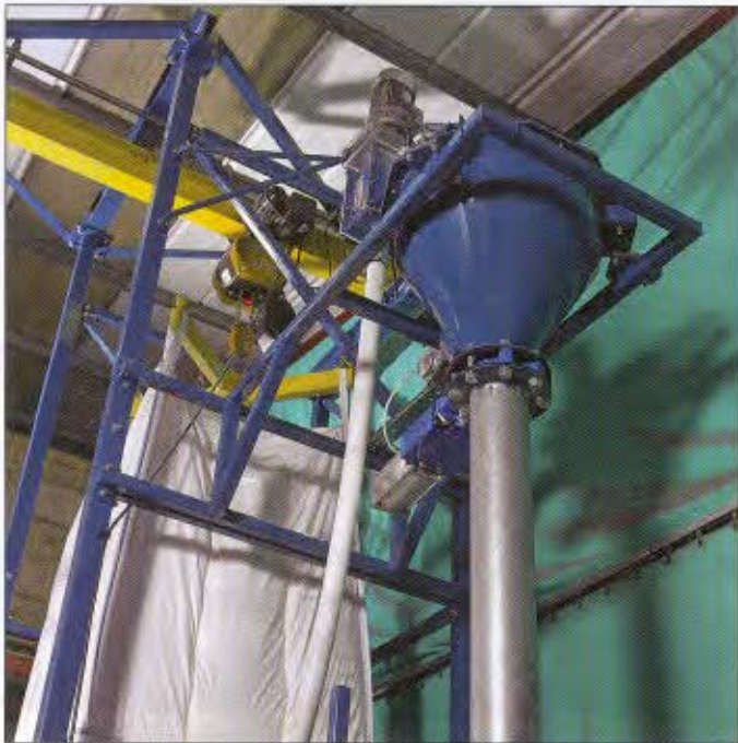
Figure 3: A flexible-screw conveyor (the narrow tube in the middle of the photo) transfers product to the weigh hopper, which is mounted on load cells that transmit gain-in-weight information to the control panel.
