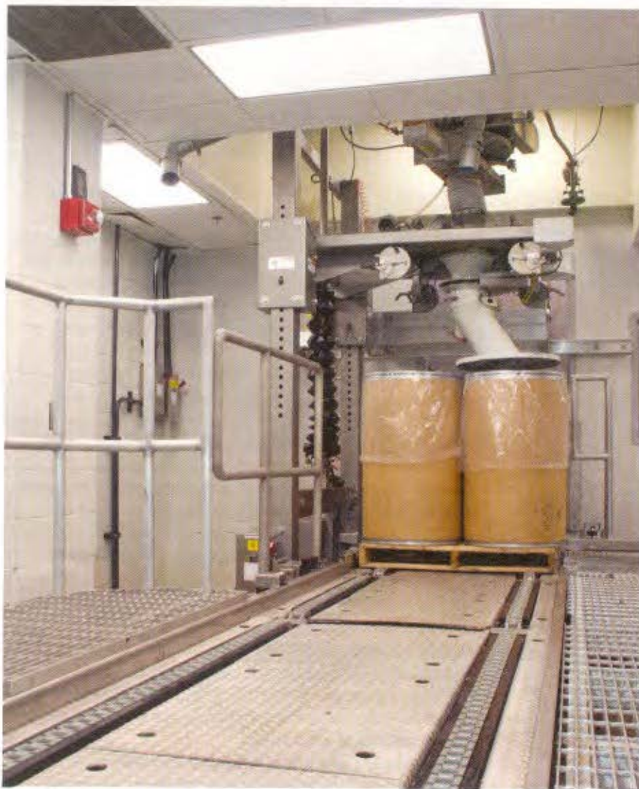
Filled drums are conveyed from loading room to shipping area
