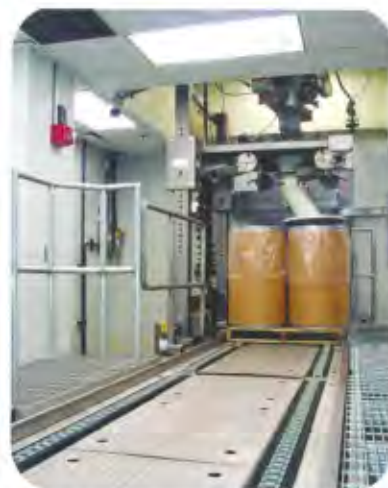
Filled drums are conveyed from loading room to shipping area
