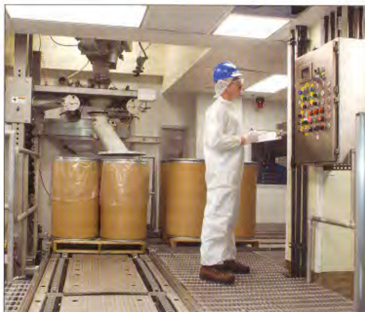
PLC communicates with weigh-filler scale to regulate product flow into each drum and shut down on reaching a pre-set weight. Four drums await filling as four are about to exit the room. System improves product output, worker safety, and quality control.
