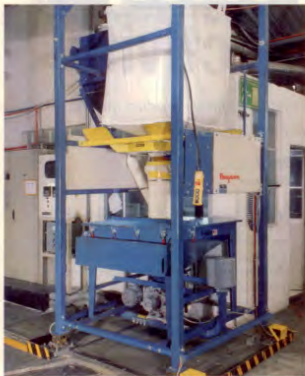
PVC from the bulk bag unloader is pneumatically transported to a 36-inch-diameter filter-receiver and hopper on the third floor of the plant. The flexible-screw conveyor empties calcium carbonate into the smaller weigh hopper. Both ingredients are then gravity fed to the mixer on the floor below.
