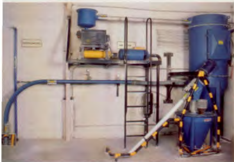
After workers load calcium carbonate additive into a bag-dump station on the second floor of the plant, a flexible-screw conveyor (at right) transports the additive 30 feet to a weigh hopper on the third floor.
