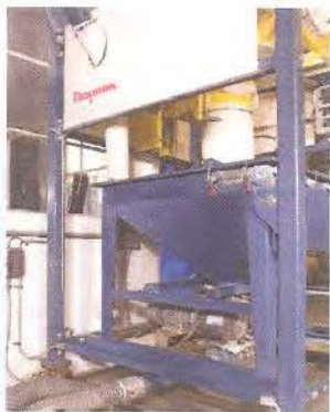
Fig. 2: Below the hopper on the bulk bag discharger frame, a drop-through rotary valve meters PVC resin into two Flexicon pneumatic conveying lines.
