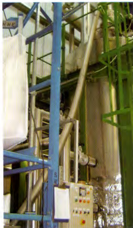
Pentaerythritol powder needed to make Midel 7131 polyol ester transformer fluid is pulled from the hopper to the discharge-transition adapter via a flexible, 20-ft.-long screw conveyor in this polyethylene tube. Next it is gravity-fed into the new 5.5-ton reactor at M & I's plant in Manchester, U.K.
