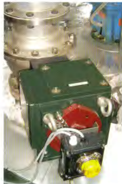
Close-up of the discharge-transition adapter that feeds bulk penta directly into M & I's reactor from the screw conveyor.
