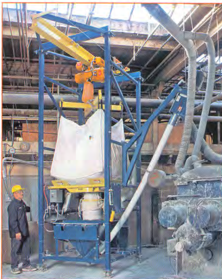
One of three bulk bag weigh batch unloading systems equipped with 226 litre capacity receiving hoppers and 114 mm diameter flexible screw conveyors, discharges powder from 1 135 kg bulk bags, transporting it under loss-of-weight control to any of three kneader-extruders. A bag tray support and hinged hopper cover allow manual additions of minor ingredients.
