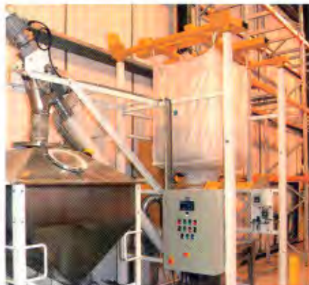
The transfer bin is mounted on a platform scale, which transmits gain-in-weight signals to a controller that runs, slows, and stops the conveyor, achieving rapid batching cycles and \pm 0.04\% batch weight accuracy.
