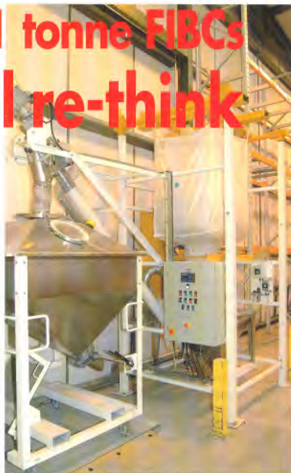
The discharge frame, control panel and intermediate hopper
