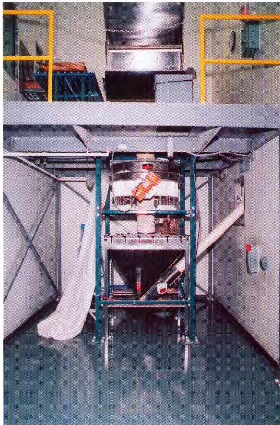
Powdered milk, emptied from bags into a bag dump station, flows through a 48-in.-diameter Kason Vibroscreen FLO-THRU circular vibratory screener into Flexicon into a Flexicon floor hopper, from which a flexible screw conveyor, at a 45-degree incline, transports the powder to a form-fill-seal machine in an adjacent room.
