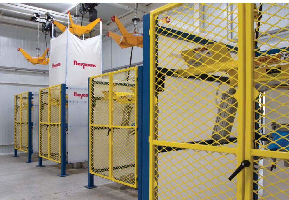
Seven Bulk-Out® model BFH-C-X half-frame bulk bag dischargers feed 70 tonnes per day to packaging machines on the floor below. An electric hoist positioned over each discharger lifts the bag onto the half frame.
