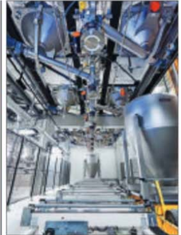
Daxner has designed and installed an advanced bakery ingredients mixing plant, featuring an automated IBC transport system, which breaks new ground in terms of powder dosing accuracy, hygiene, flexibility, reduced dust generation and minimal cross-contamination, as described on p10.
