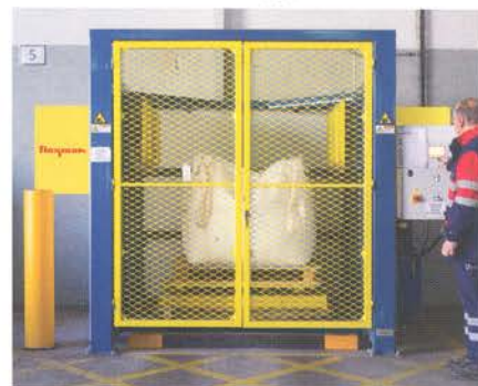
Once the safety doors are secured, the operator initiates the conditioning cycle.
