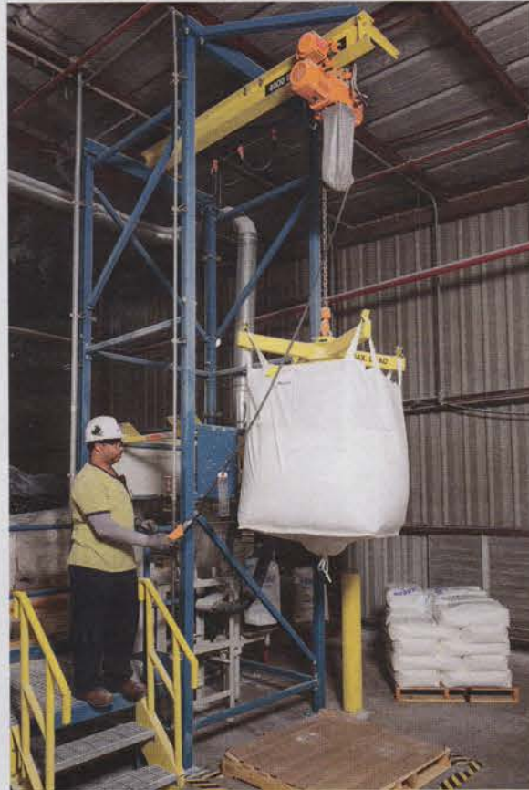
'Bulk-to-sack' system: The bulk bag is loaded into the frame using the discharger's cantilevered I-beam, electric hoist and trolley, and then gravity discharged through the telescoping tube into a filling machine for 50-lb sacks.
