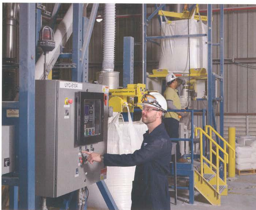
Operator in foreground initiates a bulk bag filling cycle while operator in background loads a bulk bag into the discharger frame using its electric hoist and trolley.
