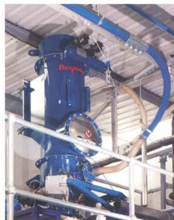
From the pneumatic line, the filter-receiver separates the silicon powder from the air stream before the powder enters the receiving hopper and is delivered to a slurry tank. A reverse pulse jet system cleans the filter cartridges at timed intervals.
