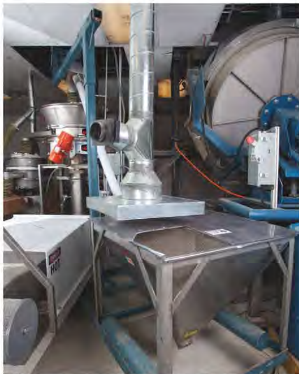
The fragile wet pellets are moved by a flexible screw conveyor to a circular fluid bed dryer, which reduces their moisture content from about 5 wt% to 0.3 wt%.
