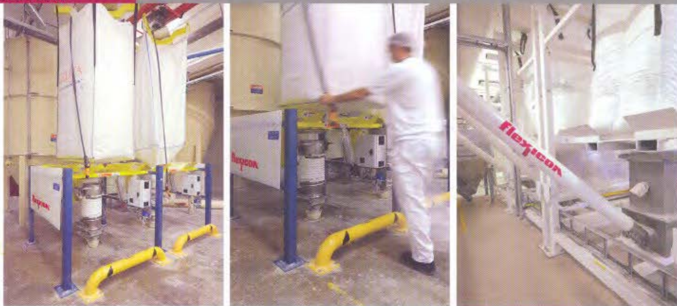
(Left and middle): Nidar AS added twin bulk bag dischargers from Flexicon to handle two types of starch in a tight space on the plant's fourth floor. (Right): Where gravity feeding of materials is not possible, the plant transfers bulk materials using bulk bag dischargers, flexible screw conveyors, rigid augers and pneumatic conveyors.
